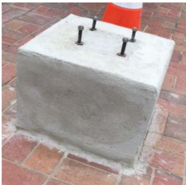
Each concrete pedestal is reinforced with rebar. They are 18" wide by 18" deep by 12" high.
